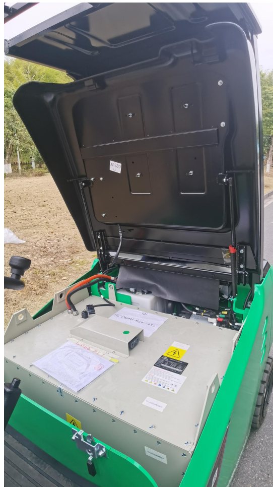
Picture 20 Battery compartment
